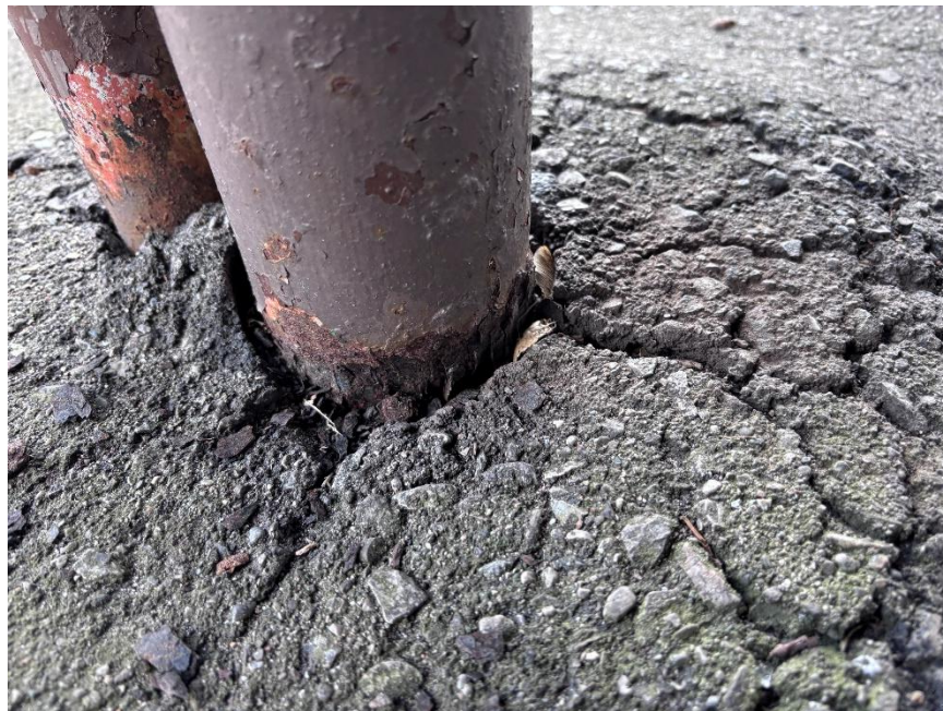
Photo 2 - Deteriorated post base and tarmac
