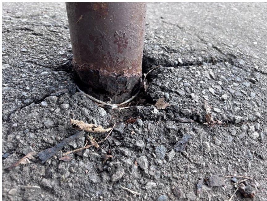
Photo 4 - Deteriorated post base and tarmac
