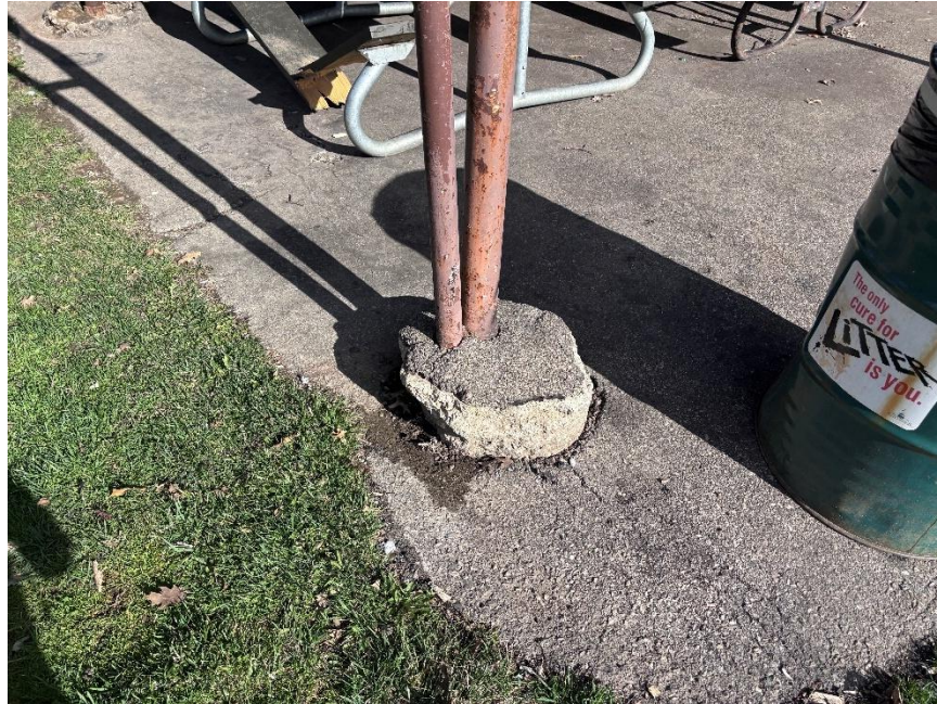
Photo 7 - Settled tarmac and exposed concrete pier
