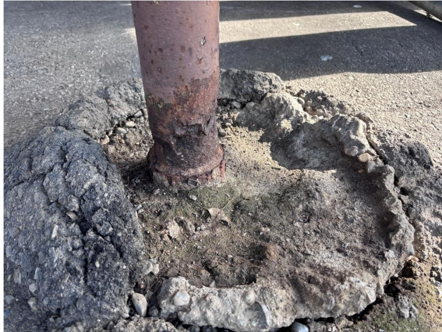
Photo 3 - Deteriorated post base and tarmac
