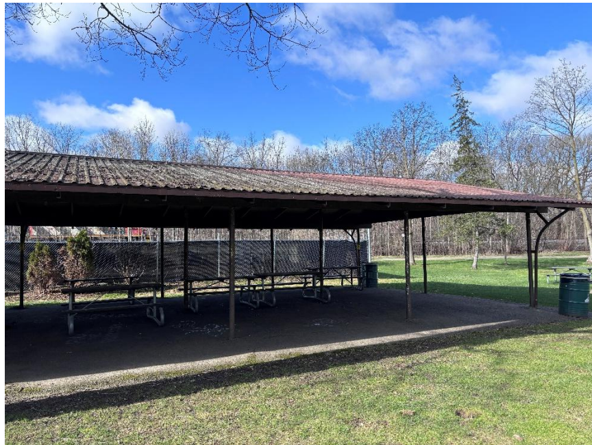
Photo 8 - Aged and weathered corrugated metal roof decking
