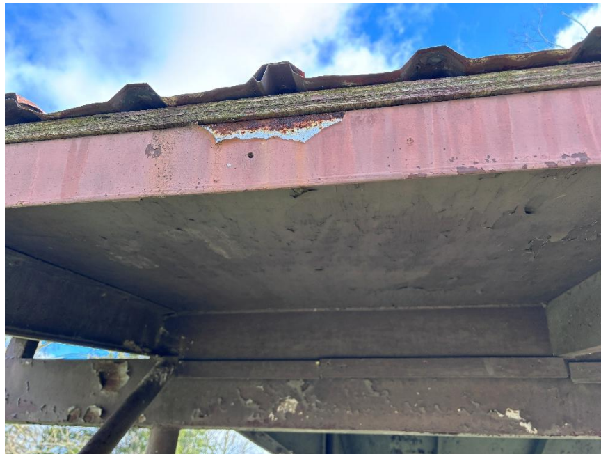
Photo 10 - Corrosion on a perimeter angle
