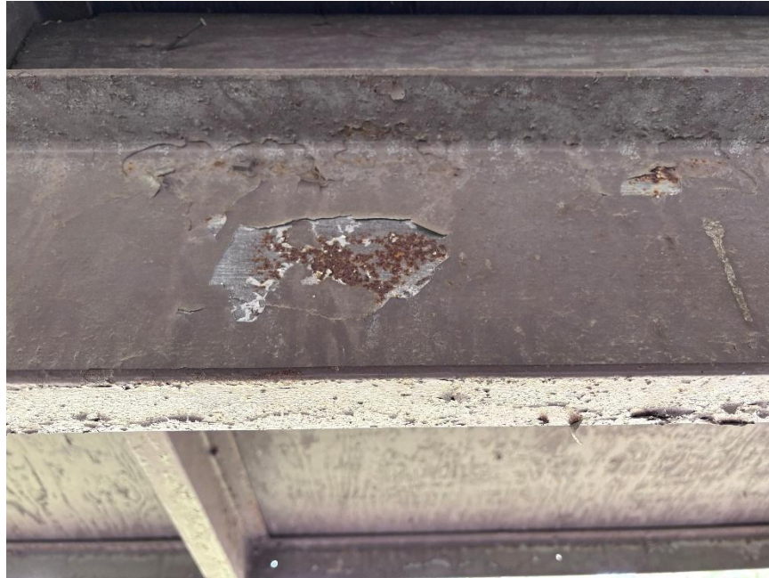
Photo 11 - Corrosion on a channel
