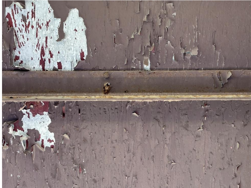
Photo 9 - Paint chipping on wood sheathing and corrosion on angle/fastener
