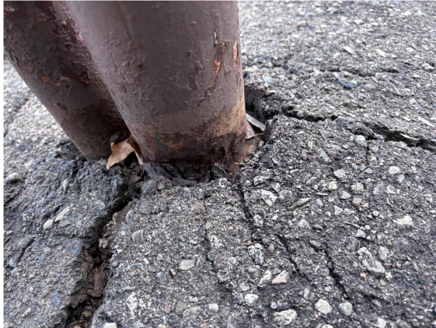
Photo 5 - Deteriorated post base and tarmac
